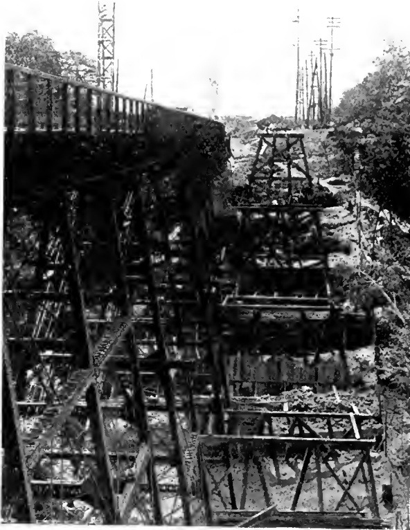
Progress of work at Reservoir Ravine bridge. The wooden trestle work will carry trains temporarily. The excavations are for new footings. The steel bridges will be removed before constructing the new bridge.
